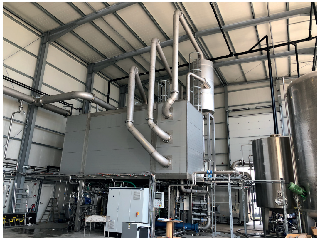
Zero liquid discharge building with the Arnold multistage vacuum evaporator
